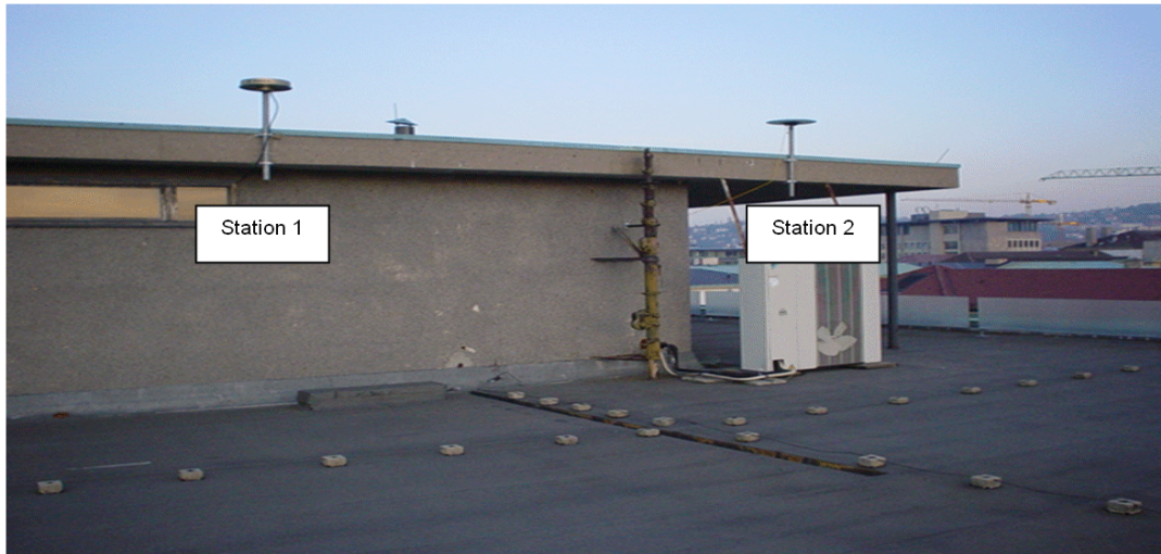
Figure 1: The antennas of station 1 and 2 on top of the institute
